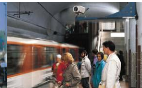
Telecommunications systems for rail applications
