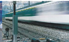
Automatic train control systems
